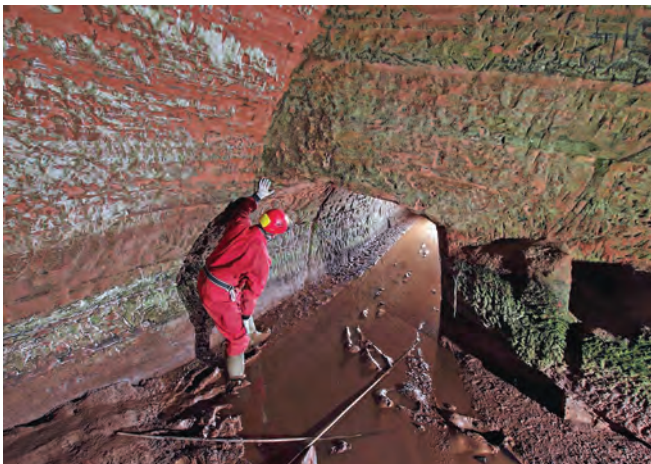
The author looking into the main tunnel (only 750 yards to go ...!). The camera position is at the right-hand corner of the railings at the end of the canal dock area. Compare this view with that of the dinghy and pontoon in 1966. It shows how much higher 'ground' level is now. Photo Ian Cooper
